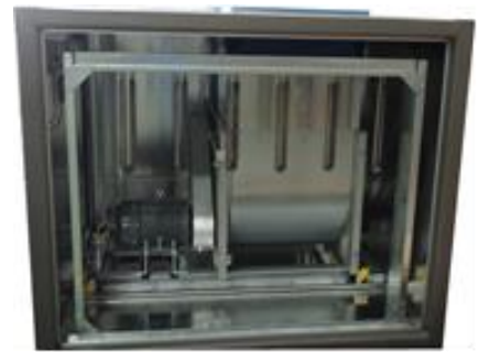
Figure 13. Electric Heater in AHU
